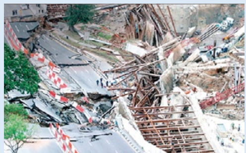
©Review of Nicolle Highway Collapse in Singapore MRT
